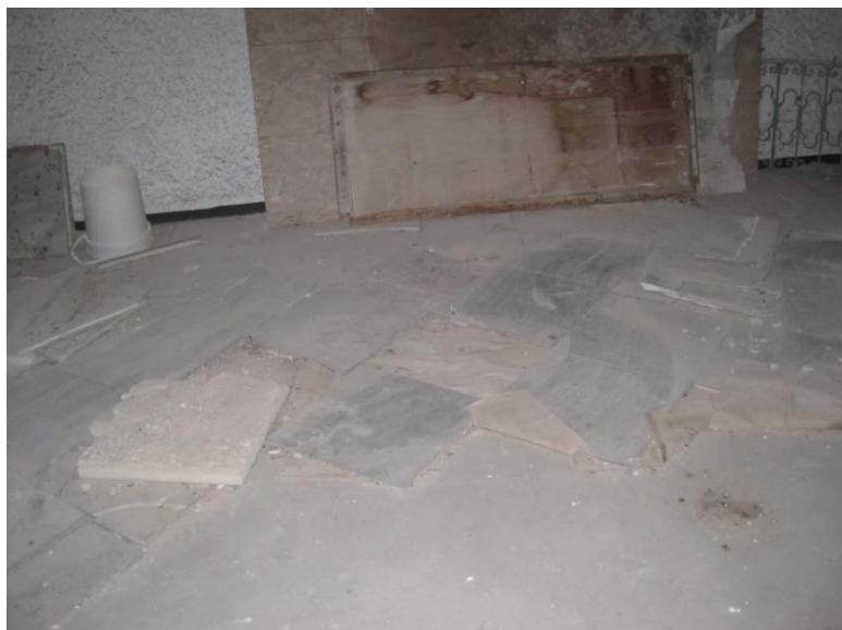
Part of the floor had to be removed in order to change the rotten wooden beams underneath them. Before removal, all the marble was documented and carefully moved to the adjoining room. They have been set temporarily in the exact order as they existed originally.
